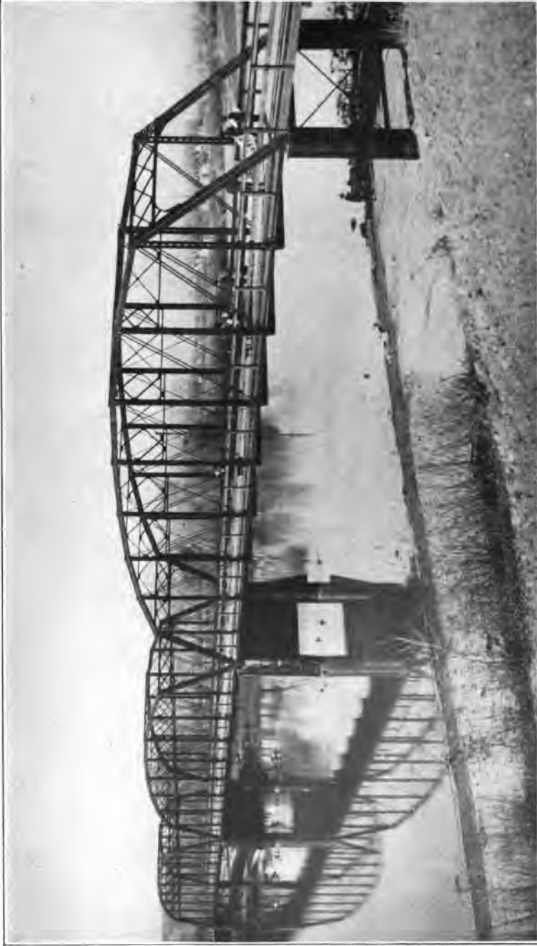
STATE HIGHWAY BRIDGE OVER GREEN RIVER AT GREENRIVER, BETWEEN EMERY AND GRAND COUNTIES, MIDLAND BRIDGE COMPANY, CONTRACTOR.
